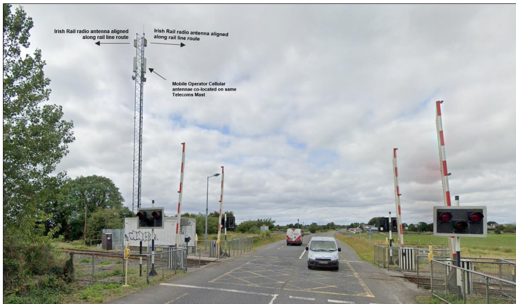
Figure 3. Example of GSM-R Train Radio installation using Directional Sector Antennas
