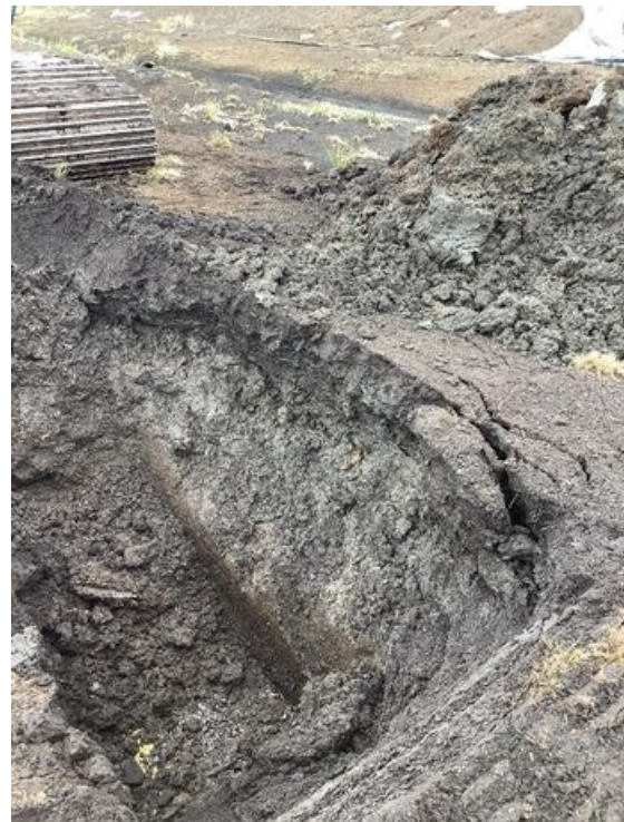
Plate 16: TP8 after collapse of peat
