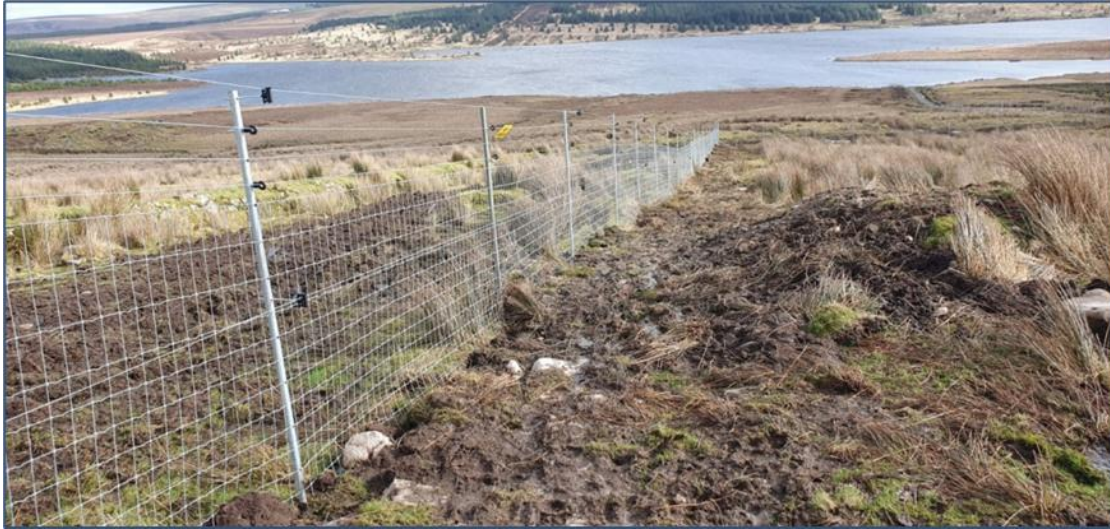
Plate 3- 1 Example predator-proof fencing broadly in-line with proposed specifications (for illustrative purposes only) .
