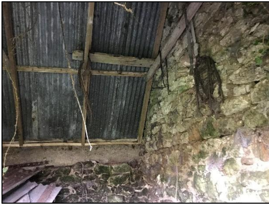
Plate 4-5 Interior of stone shed showing galvanised roof, timber framing, stonework and influx of light
