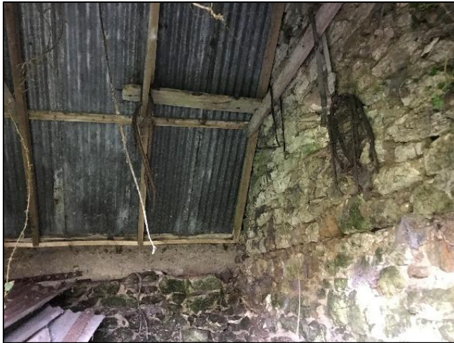
Plate 3-5 Interior of stone shed showing galvanised roof, timber framing, stonework and influx of light
