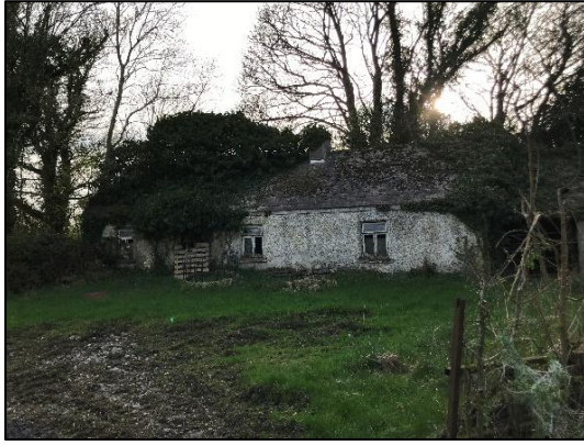
Plate 3-1 Exterior of house showing open windows and ivy overgrowth
